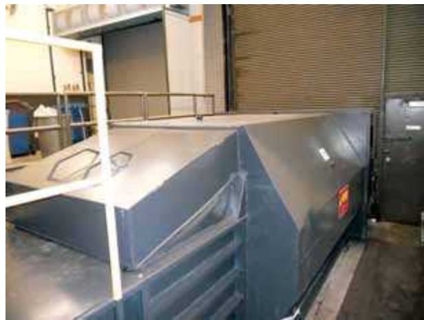
Large rubbish container in a protected room.
