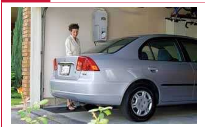
A residential CNG refueling system. (Courtesy of cleanenergyfuels.com)
