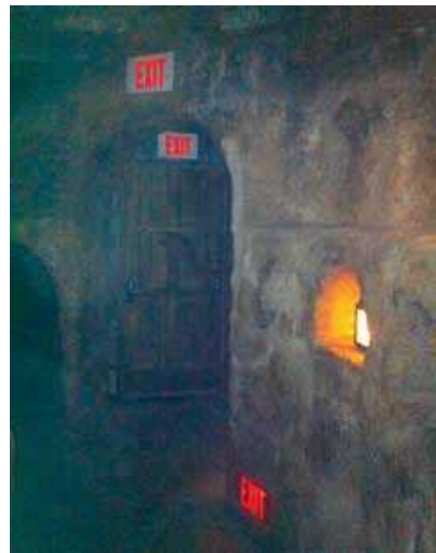
Floor proximity exit sign in special amusement building.
