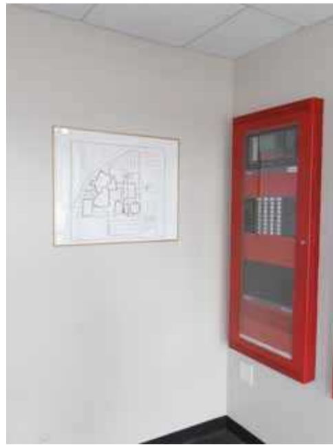
Alarm system annunciator panel.
