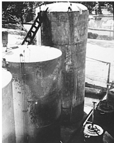
Damage to tanks caused by inadequate normal outflow venting capacity.
