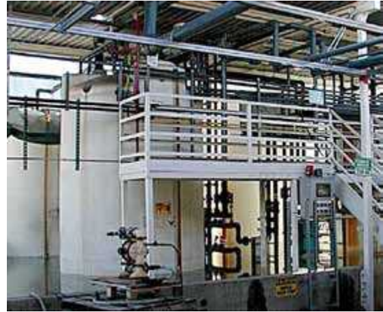
A typical chemical process plant.
