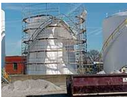
Damage to tanks caused by inadequate normal inflow venting capacity.
