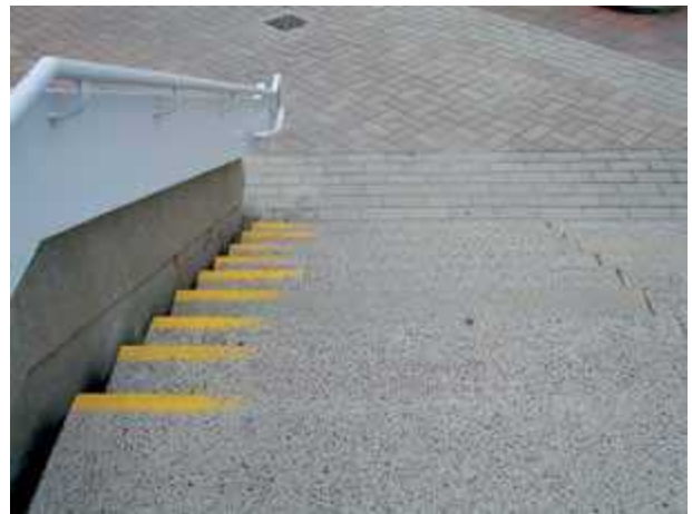
Stair tread marking worn away so as to make tread location imperceptible. (Photo courtesy of Jake Pauls)
