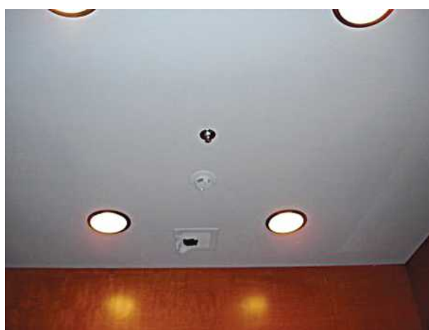
Automatic sprinklers on a production set.
