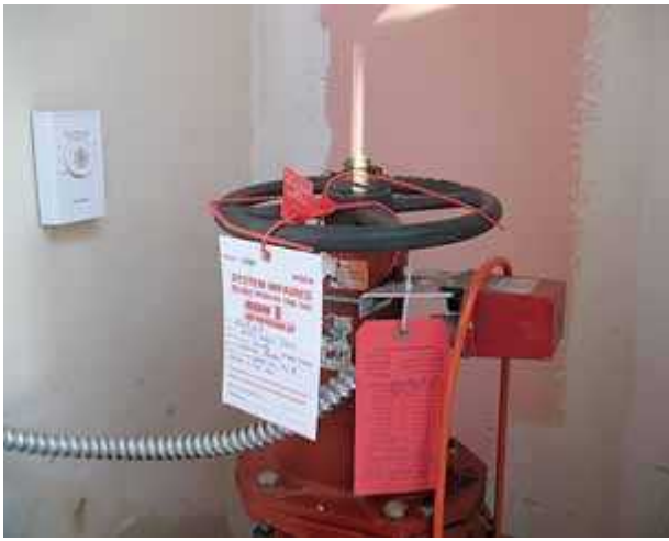
Example of an impaired system tag. (Courtesy of Byron Blake and SimplexGrinnell)
