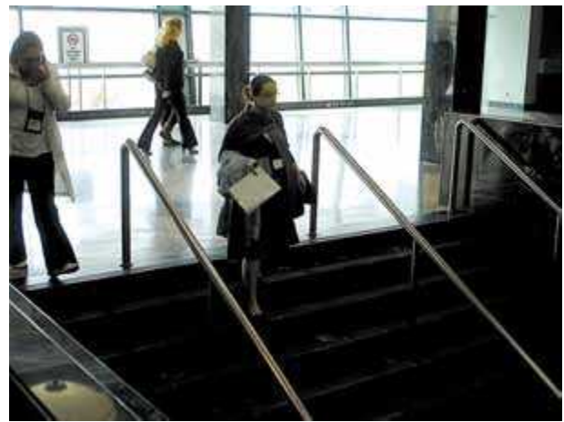
Poorly lit interior stair near brightly lit window space. (Courtesy of Jake Pauls)
