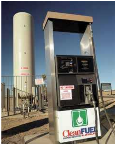
Typical propane storage and dispensing system for fueling vehicles. (Photo: Warren Gretz; Courtesy of DOE/NERL)
