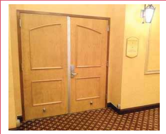
Automatic-closing door in closed position.
