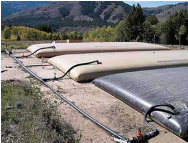
Portable storage tanks as an alternative source of water. (Courtesy of National Park Service)
