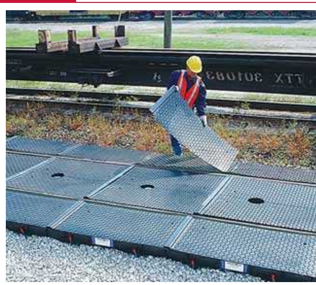
Rail tank car loading/unloading position being retrofitted with spill retention capability. (Courtesy of UltraTech International, Inc.)
