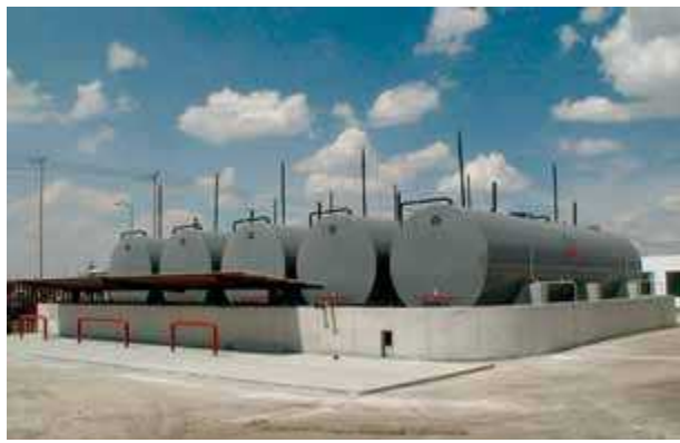
Horizontal aboveground atmospheric storage tanks.
