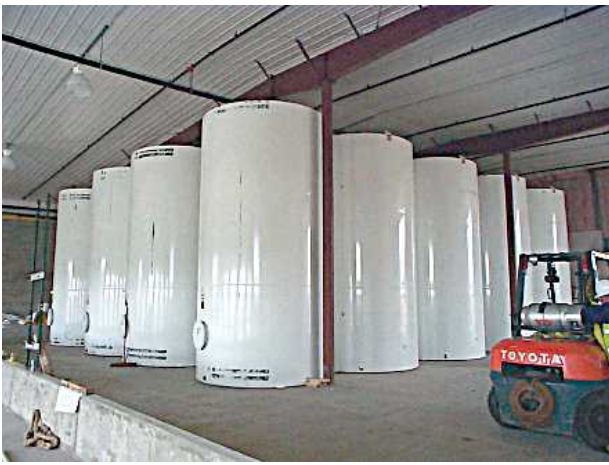
Storage tank installation inside a building.
