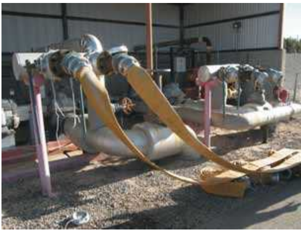
Outdoor fire pump installation. (Courtesy of Aon Fire Protection Engineering)
