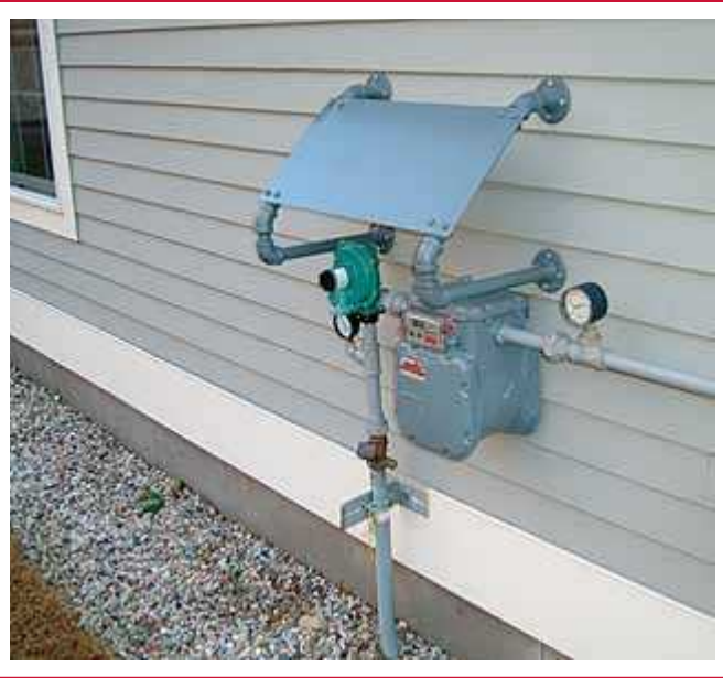
A method of meter protection in heavy snow areas. (Courtesy of Dead River Company)
