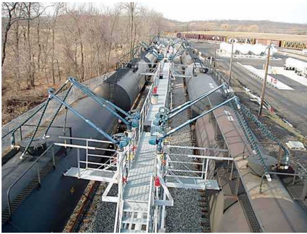
Tank car loading/unloading facility. Note the swing arms connected to the tank car dome. (Courtesy of Eastern Propane Corp.)
