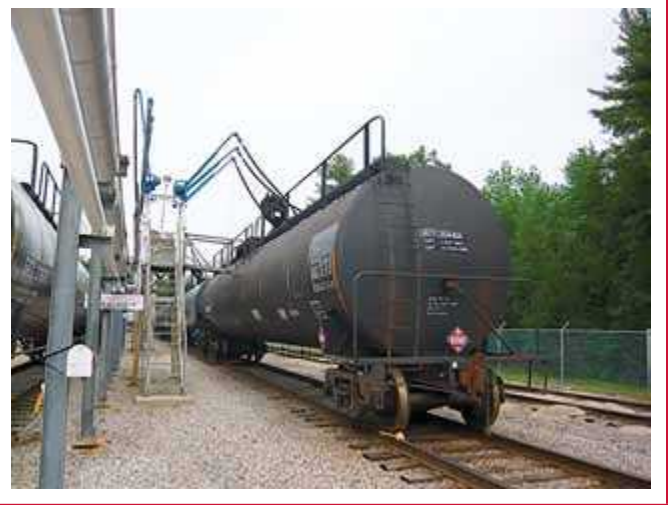
Railcar unloading tower. (Courtesy of Eastern Propane Gas Inc.)
