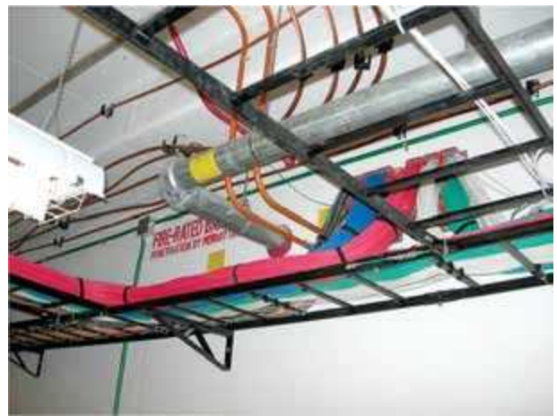
Cable penetrations through a fire barrier.
