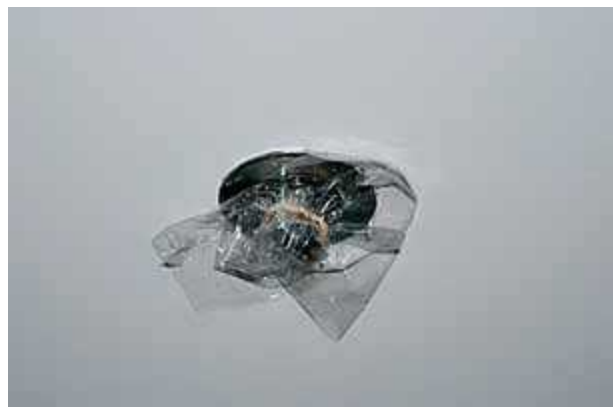
Sprinkler protected from overspray with a cellophane bag.
