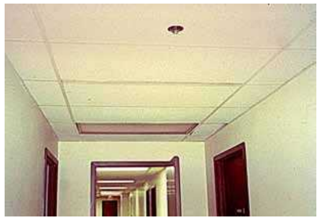
Retrofitted cross-corridor door that affects sprinkler spacing.
