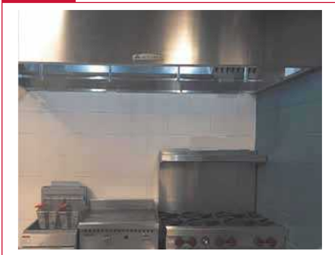
Hood suppression system. (Courtesy of Tyco Fire Protection Products)
