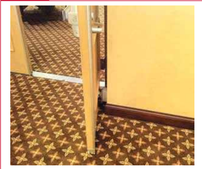
Automatic-closing door in open position.
