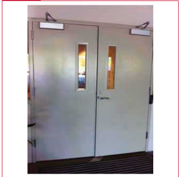
Pair of swing fire doors with vertical clearance between the doors in excess of \frac{1}{8} in. (3.18 mm). (Courtesy of the Door Security & Safety Foundation, Door and Hardware Institute)
