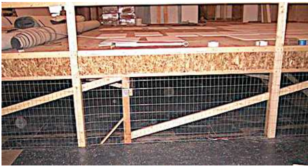
Platform protected from storage being placed underneath.
