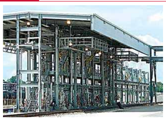
Loading rack protected with a canopy. (Courtesy of Carbis, Inc.)
