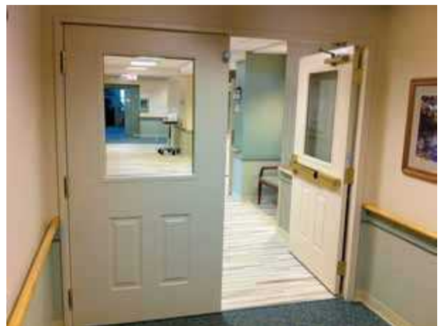
Cross-corridor smoke barrier doors, which are part of the defend-in-place protection strategy.
