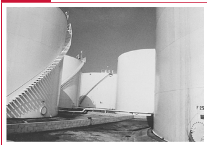
Intermediate dikes around tanks.
