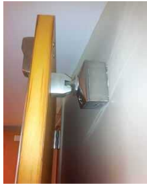
Hold-open mechanism on automatic-closing door.
