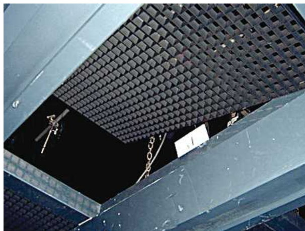
Smoke detector above a grid ceiling.
