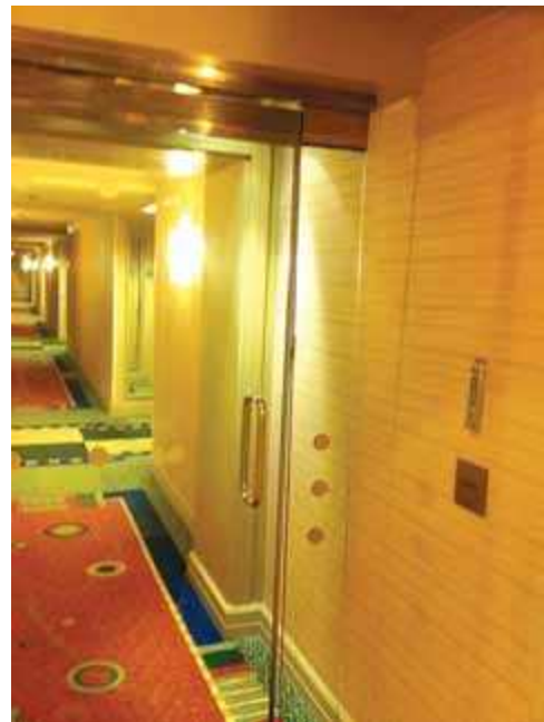
Non-egress side of sensor-release of electrical locking system door assembly.
