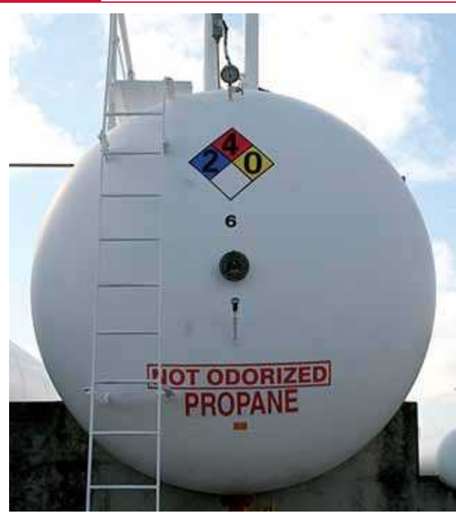
ASME container marked “NOT ODORIZED.” (Courtesy of National Propane Gas Association)
