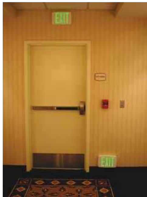
Floor proximity EXIT sign. (Courtesy of Jake Pauls)
