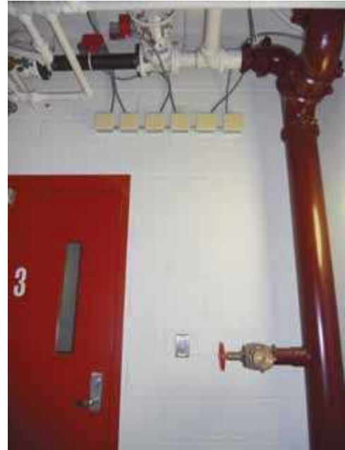
Typical combination sprinkler/standpipe system with a 2½ in. (64 mm) fire department valve.
