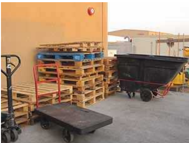
FDC obstructed and inaccessible due to exterior storage. (Courtesy of Byron Blake and SimplexGrinnell)
