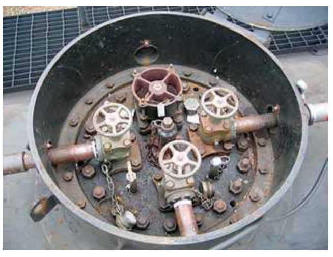
Close-up of tank car dome. (Courtesy of Eastern Propane Corp.)
