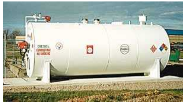
Typical secondary containment tank. (Courtesy of Modern Welding Co.)
