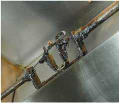
Fusible link requiring replacement.
