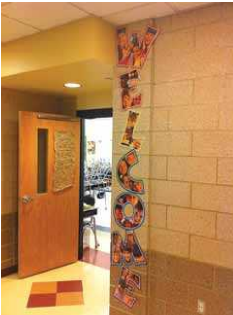
Classroom door swinging into recessed pocket in corridor.
