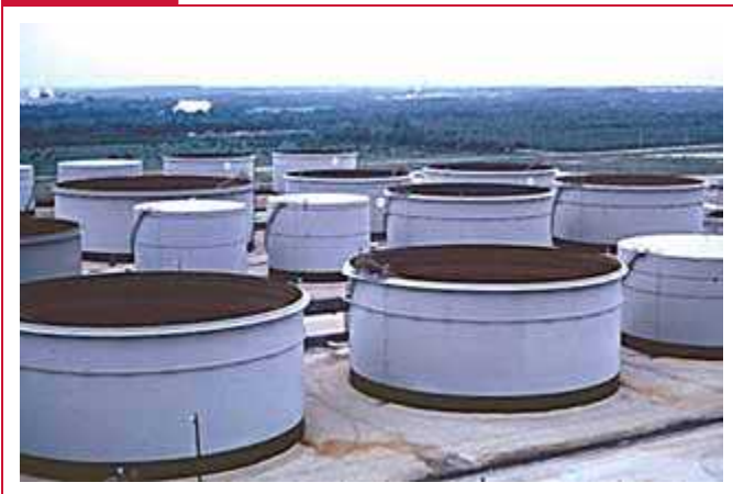
Open-top floating roof tanks.
