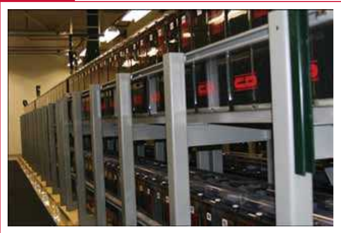
Stationary storage battery system. (Courtesy of Applied Power Services, LLC)
