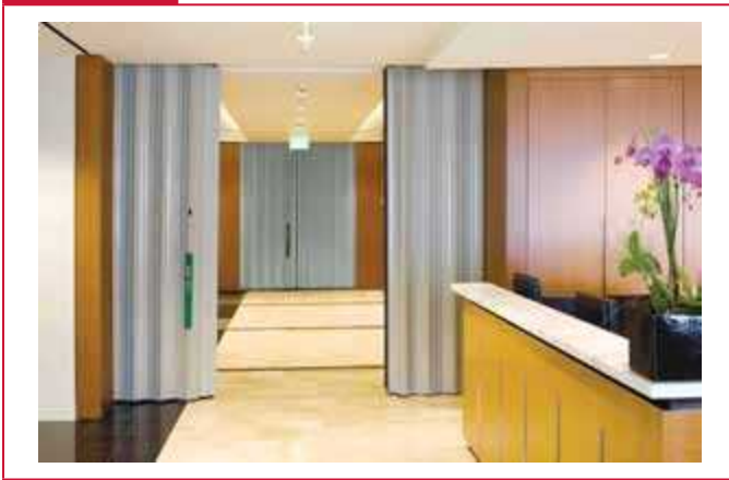
Special-purpose horizontally sliding accordion door assembly addressed by 14.5.10. (Photo courtesy of Won-Door Corp.)
