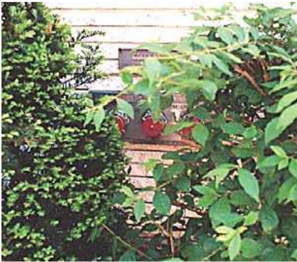
FDC obstructed by shrubbery.
