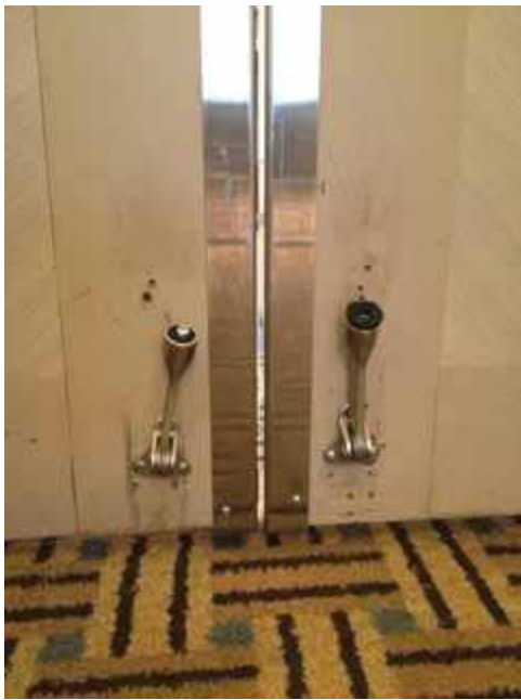
Pair of swing fire doors with noncompliant vertical clearance.
