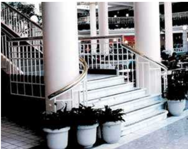
Potted plants prevent access to required handrails. (Courtesy of Jake Pauls)
