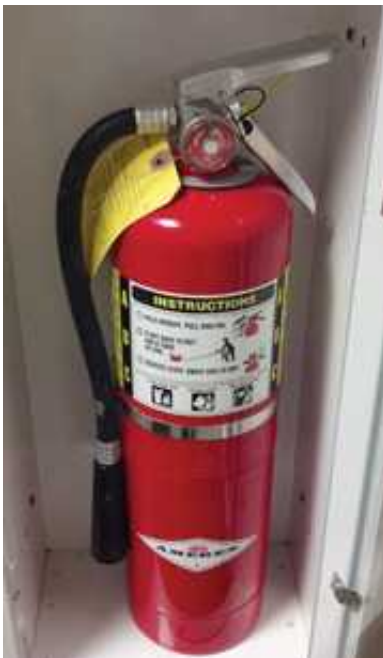
Inspection and maintenance tags on a cabinet-mounted extinguisher.
