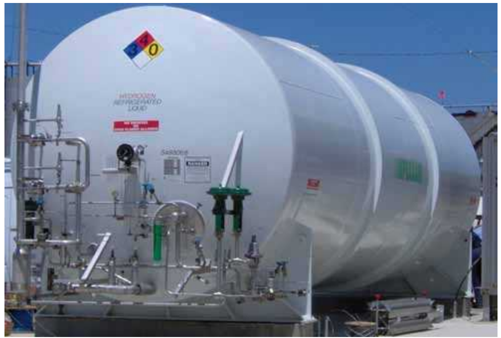
Signage on cryogenic fluid container.
