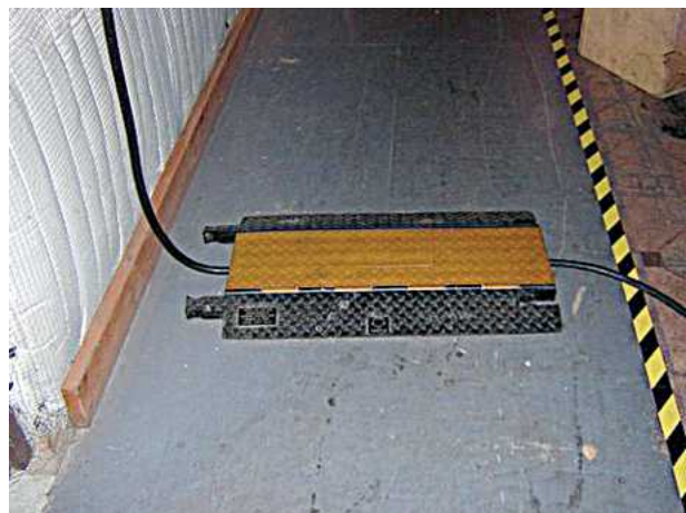
Example of properly protected cables in an aisle.
