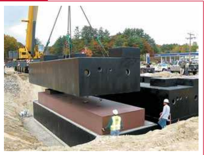
Vault and its storage tank being installed at a service station site. (Courtesy of Core Engineered Solutions, Inc.)
