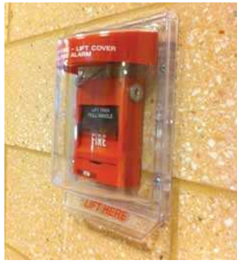
Manual fire alarm box with protective cover.
