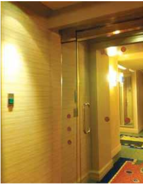
Circular decals that call attention to glass door in corridor egress path.
