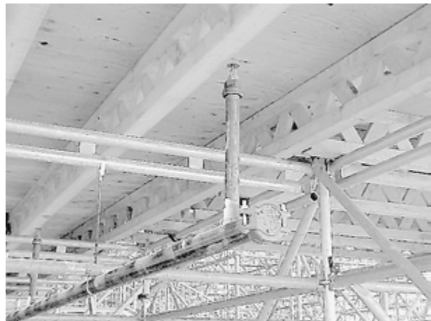
Sprinklers installed under a grandstand.
