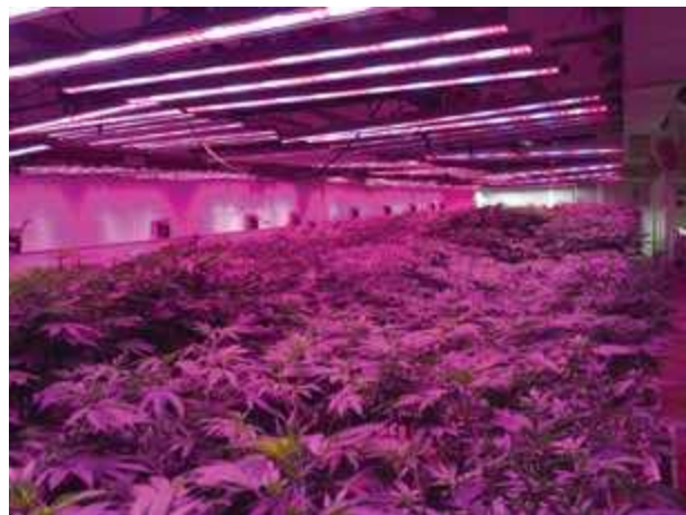
Complex arrangement of light fixtures in marijuana growing area.
