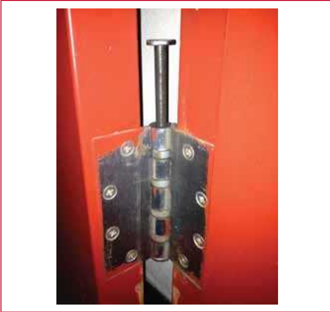
Fire door with hinge pin not secured in proper position.
