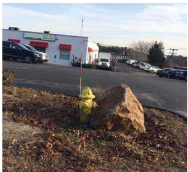
Fire hydrant without proper clearance maintained.
