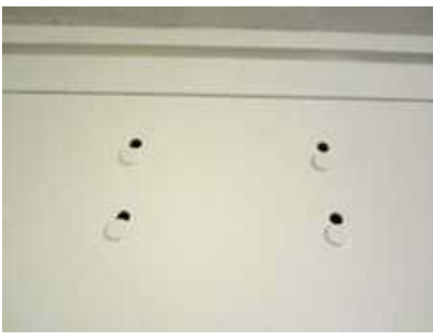
Fire door with an extra set of holes for installation of closing device. (Courtesy of Lori Greene)
