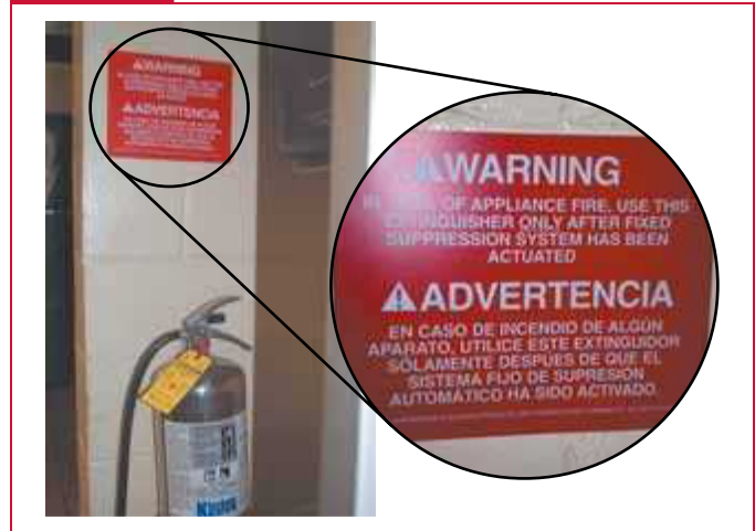
Required placard located directly above the fire extinguisher.
