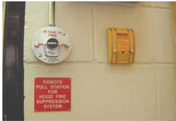
Example of a properly located manual pull station.
