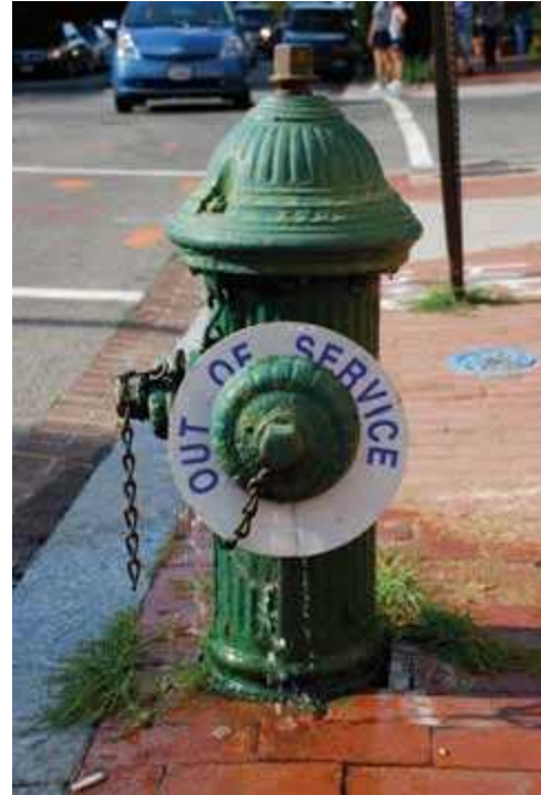
Fire hydrant with out of service indicator.
