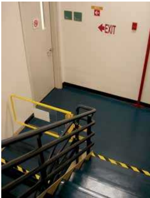
Interruption of exit stair at LED. (Courtesy of Jake Pauls)
