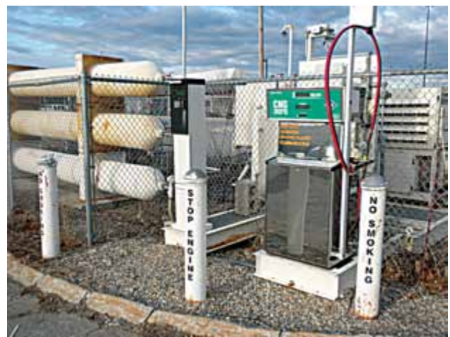
EXHIBIT 500.3 A CNG filling station, which is a Class I location.
