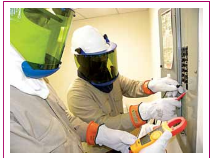
EXHIBIT 110.9 Workers clothed in personal protective equipment (PPE) appropriate for the hazard involved. (Courtesy of KTR Associates/ ArcFlashPPE.com)
