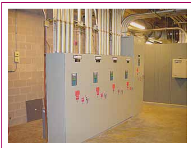
EXHIBIT 110.17 An equipment location that is free of storage to allow the equipment to be worked on safely. (Courtesy of the International Association of Electrical Inspectors)
