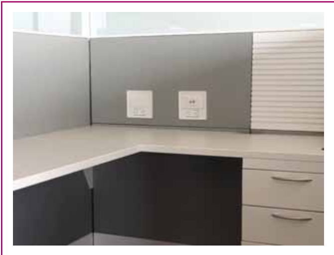
EXHIBIT 605.1 Example of a fixed-type office partition where the branch-circuit wiring is run inside the partition.
