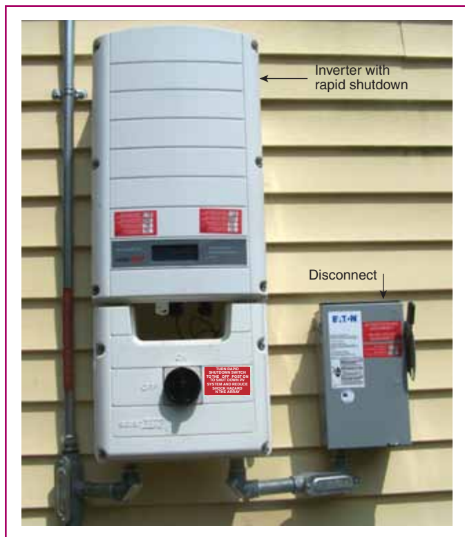
EXHIBIT 690.3 An interactive inverter. (Inverter courtesy of SolarEdge Technologies; Photo courtesy of Michael and Diane Mello)
