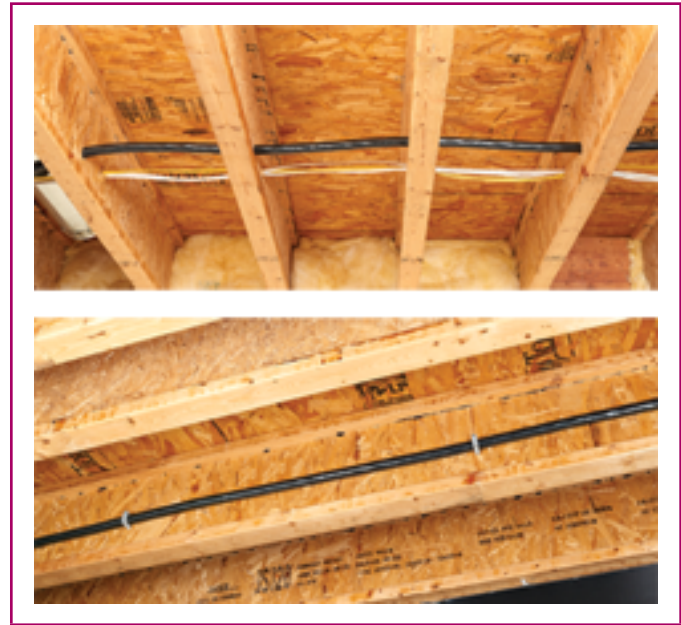
EXHIBIT 336.1 TC-ER cable installed in accordance with Part II of Article 334. (Courtesy of Generac Power Systems, Inc.)
