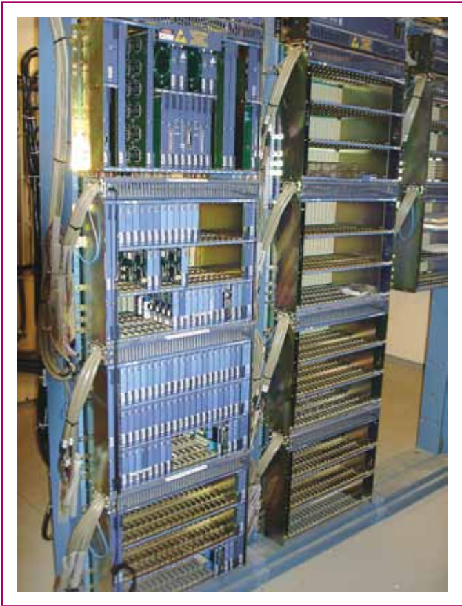
EXHIBIT 800.1 A private automatic branch exchange, which is one part of telecommunications equipment.
