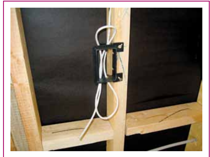
EXHIBIT 800.5 Communications outlet provision installed at “rough-in.” (Courtesy of the International Association of Electrical Inspectors)
