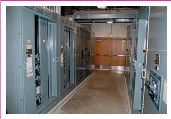
EXHIBIT 110.23 An installation of large equipment showing one of the required exits. (Courtesy of the International Association of Electrical Inspectors)
