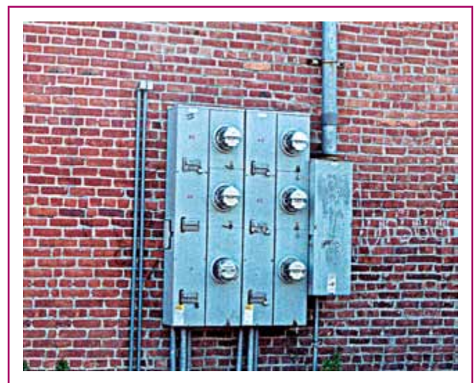
EXHIBIT 230.23 A service equipment enclosure that groups six service disconnecting means.
