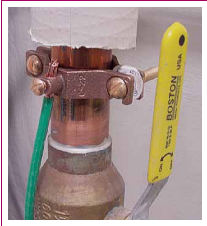
EXHIBIT 250.31 An application of a listed ground clamp.
