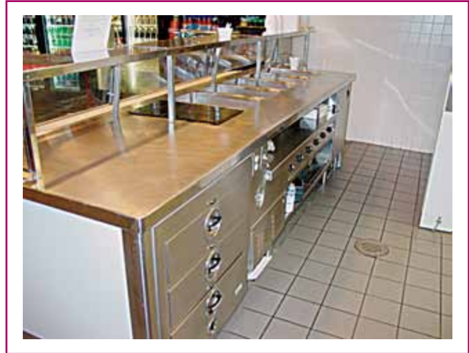
EXHIBIT 220.7 Electrically powered cooking/heating appliance with thermostatic control in a commercial kitchen. (Courtesy of the International Association of Electrical Inspectors)
