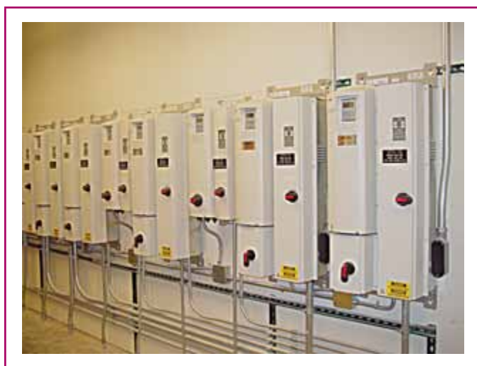
EXHIBIT 430.22 Adjustable-speed drives for air-handling units provide significant power savings for fan appliances. (Courtesy of International Association of Electrical Inspectors)
