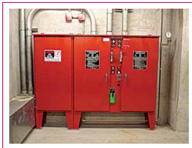
EXHIBIT 695.6 Listed fire pump controller and power transfer switch.
