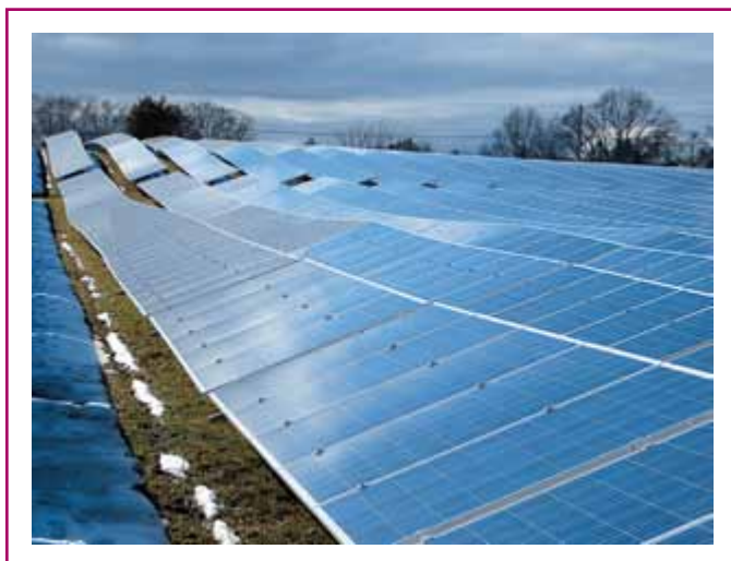
EXHIBIT 690.1 A PV array. (Courtesy of Solar Design Associates, LLC)
