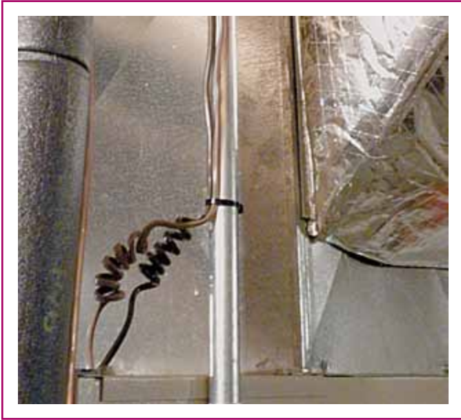
EXHIBIT 300.12 Raceway used to support Class 2 thermostat cables.
