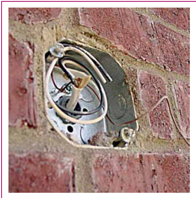
EXHIBIT 314.7 A galvanized box installed in a brick wall. (Courtesy of the International Association of Electrical Inspectors)
