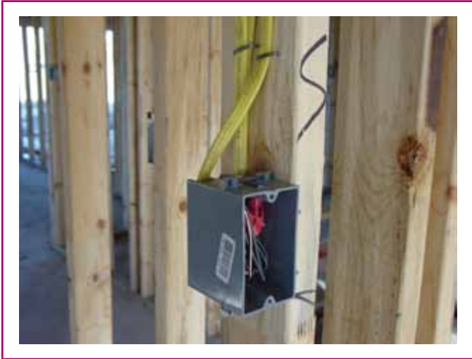
EXHIBIT 314.5 Installation of a single gang outlet with cables securely fastened within 8 inches of the box. (Courtesy of the International Association of Electrical Inspectors)
