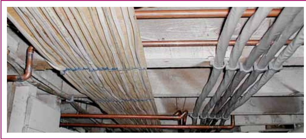
EXHIBIT 334.1 Nonmetallic-sheathed cables and Type SE cables installed in an unfinished basement or crawl space.
