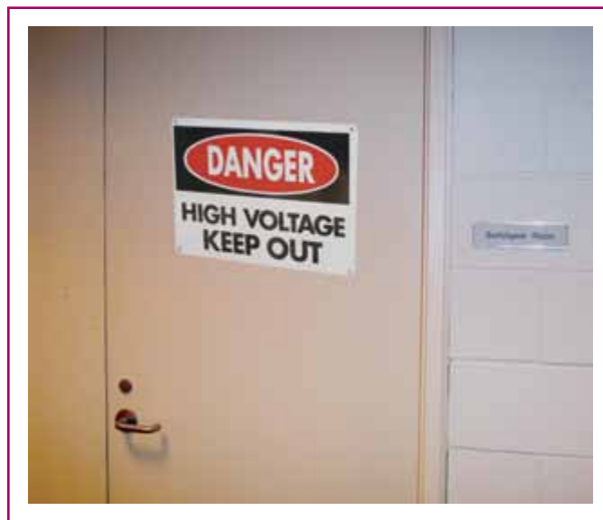
EXHIBIT 100.3 A warning sign on a locked electrical equipment door.
