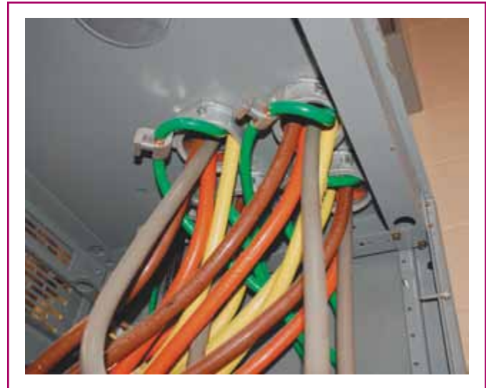
EXHIBIT 215.3 Different colors being used to identify each ungrounded line or phase conductor of a nominal voltage system.
