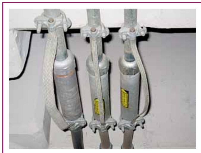
EXHIBIT 100.5 Equipment bonding jumpers installed to maintain electrical continuity around conduit expansion fittings. (Courtesy of the International Association of Electrical Inspectors)
