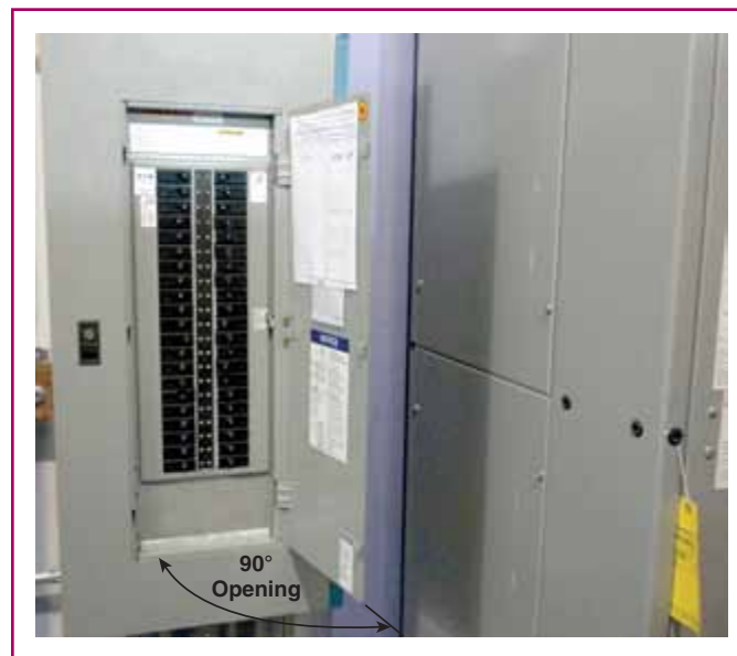
EXHIBIT 110.16 A full 90-degree opening of an equipment door in order to ensure a safe working approach.
