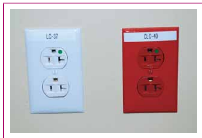
EXHIBIT 517.4 A receptacle from the normal system (left) and the critical branch (right). Note the label that indicates the panelboard and the circuit number. (Courtesy of the International Association of Electrical Inspectors)
