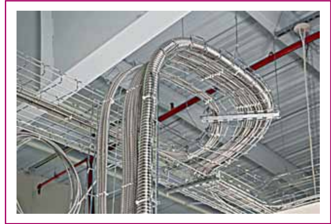
EXHIBIT 392.1 MC cable installed in a cable tray. (Courtesy of Legrand®)
