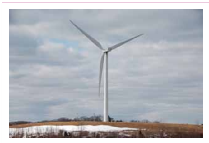
EXHIBIT 694.1 A wind electric system consisting of a single wind turbine.
