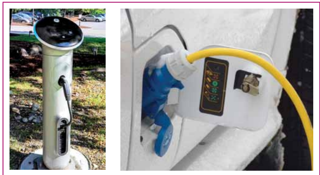
EXHIBIT 625.2 EV supply equipment (left) and a connection to a vehicle (right).
