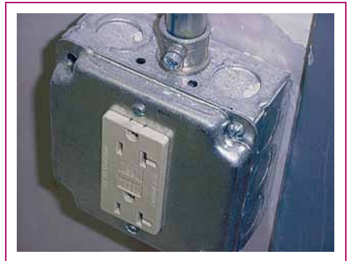
EXHIBIT 250.50 An example of a cover-mounted receptacle attached to a surface box where a bonding jumper from the grounded metal box to the receptacle is not required.
