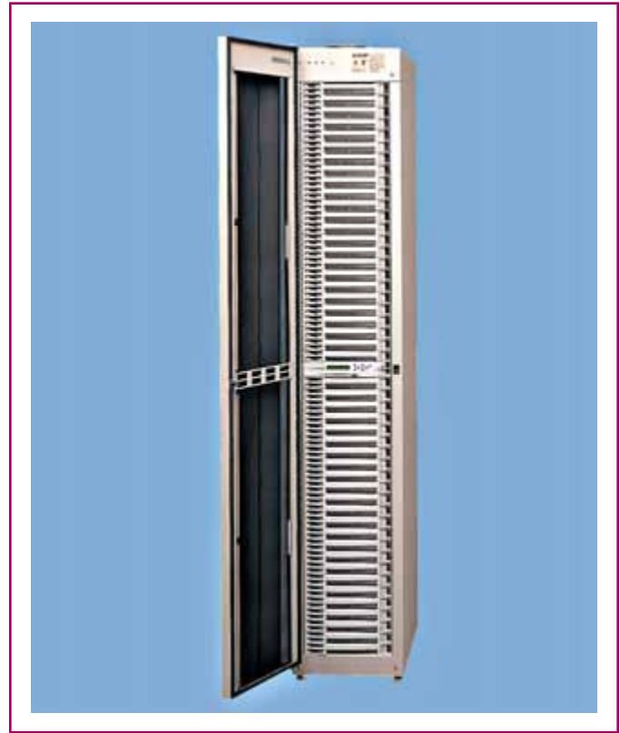
EXHIBIT 520.3 A typical high-density digital SCR dimmer switchboard. (Courtesy of Electronic Theatre Controls, Inc.)
