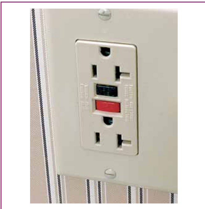
EXHIBIT 210.8 A 15-ampere duplex receptacle with integral GFCI that also protects downstream loads.
