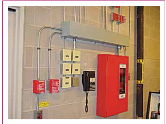
EXHIBIT 760.1 Typical fire alarm control unit. (Courtesy of the International Association of Electrical Inspectors)
