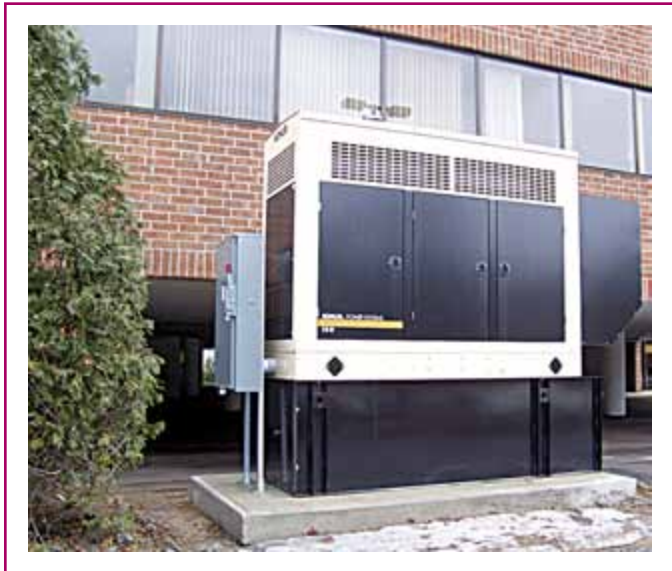
EXHIBIT 225.6 Disconnecting means for alternate source feeder supplying emergency, legally required standby, or optional standby loads or a combination of the three.
