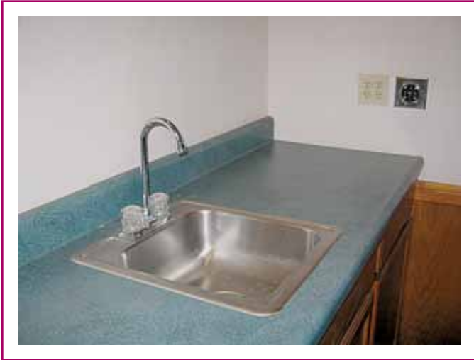
EXHIBIT 210.16 GFCI protection required for single-phase, 125-volt, and 250-volt, 15-ampere duplex receptacles installed within 6 feet of a sink if the receptacles are rated 50 amperes or less.
