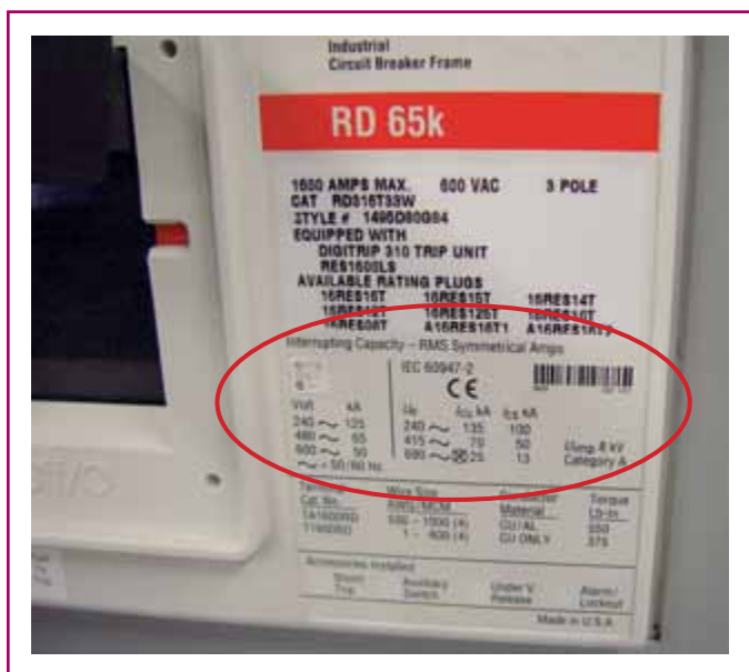
EXHIBIT 100.12 Interrupting ratings information on the label of a 1600-ampere frame circuit breaker.
