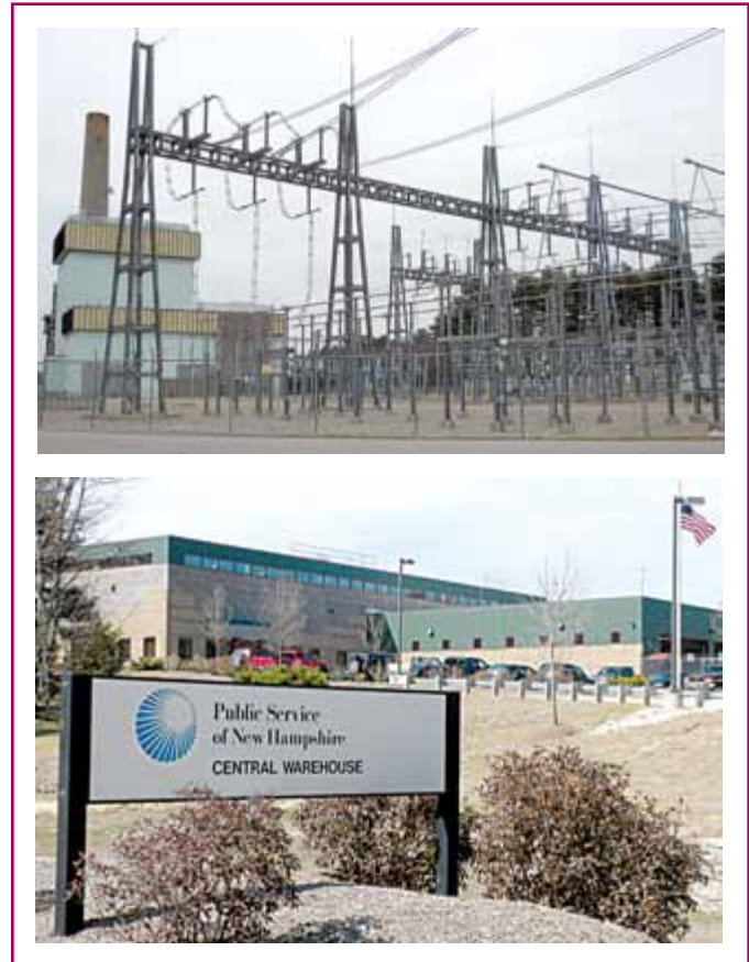
EXHIBIT 90.1 A conventional generating plant, which is governed by the National Electrical Safety Code (top); a support facility that is subject to NEC requirements (bottom).
