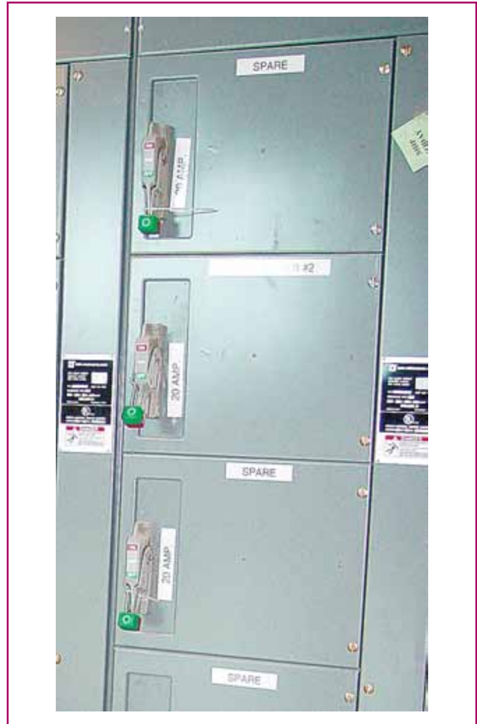
EXHIBIT 90.2 A switchboard with spare circuit breakers installed to facilitate future growth. (Courtesy of the International Association of Electrical Inspectors)
