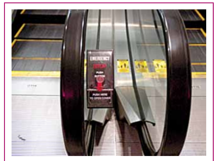
EXHIBIT 620.5 The emergency stop button installed at the escalator location is not considered to be the required disconnecting means.
