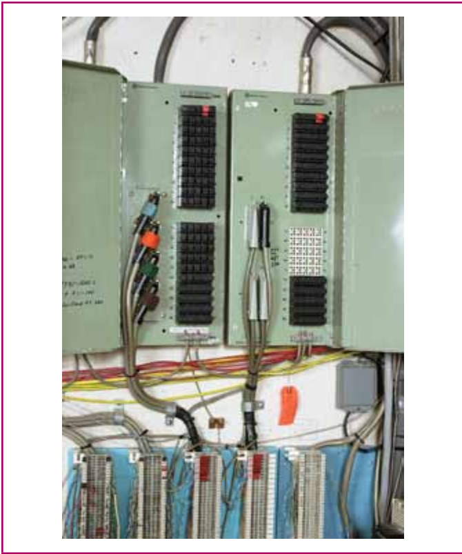
EXHIBIT 800.3 A primary protector unit installed in a commercial building that is the interface to the outside plant cable.
