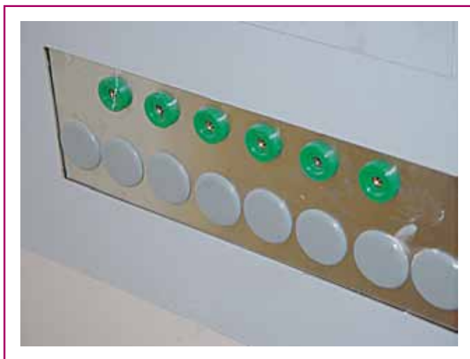
EXHIBIT 517.6 A patient equipment grounding point. (Courtesy of the International Association of Electrical Inspectors)
