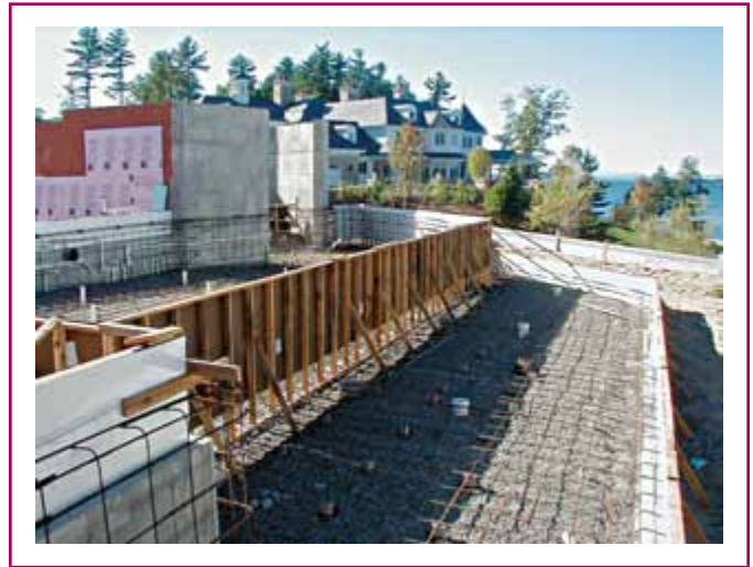
EXHIBIT 680.8 A poured-concrete pool with structural reinforcing steel that serves as the pool shell bonding grid.
