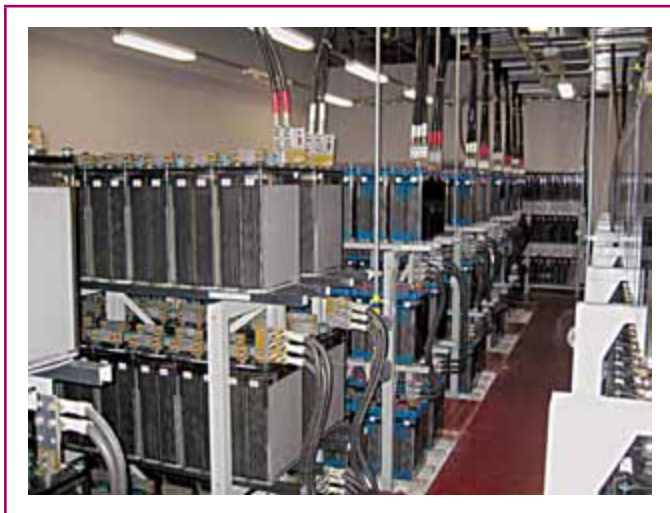
EXHIBIT 480.1 A well-arranged battery room with batteries installed on corrosion-resistant racks. (Courtesy of the International Association of Electrical Inspectors)
