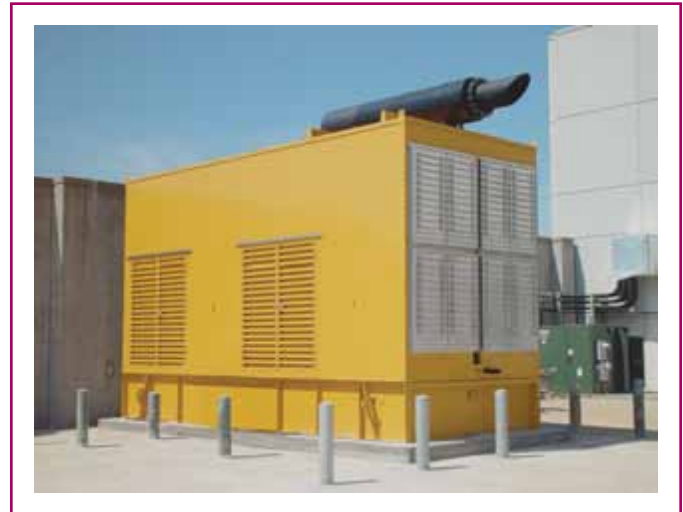
EXHIBIT 700.7 Alternate source of power in a heated and secure enclosure that is located in an area not subject to flooding. (Courtesy of the International Association of Electrical Inspectors)
