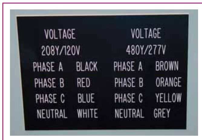
EXHIBIT 200.3 A label on a piece of equipment containing conductors of two nominal voltage systems that provides the required identification of the two systems.
