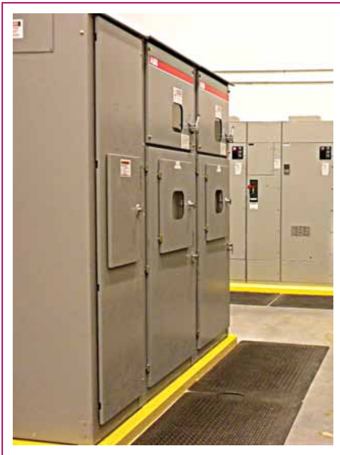
EXHIBIT 110.28 Medium voltage switchgear.
