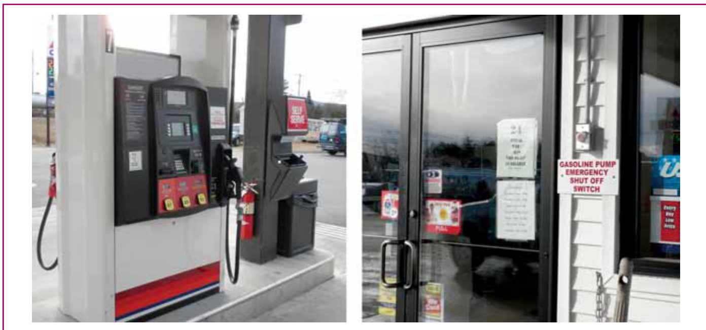
EXHIBIT 514.6 A self-service dispensing island (left) and associated emergency disconnecting means (right).
