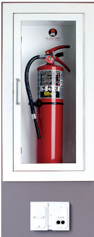
Fire Extinguisher Monitored by Fire Extinguisher Monitoring Device. (Source: en-Gauge, Inc., Rockland, MA)
