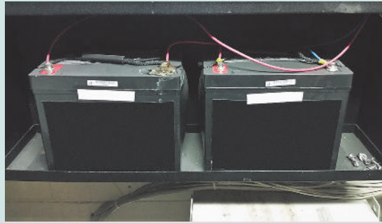
Batteries with Corrosion and Case Swelling. (Courtesy of Norel Service Company, Inc., Waltham, MA)
