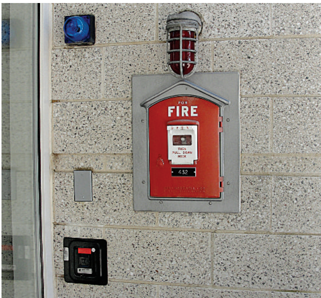
Auxiliary Alarm Box.
