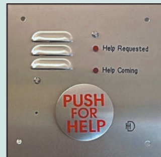
Area of Refuge Station Used for Emergency Communications. (Courtesy of Housing Devices, Inc., Medford, MA)
