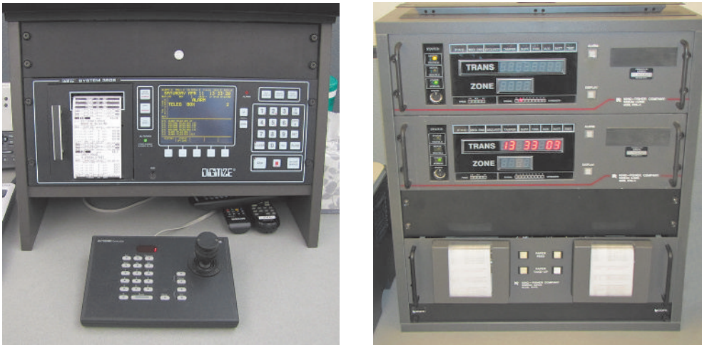
Alarm Processing Equipment. Left: wired equipment; right: wireless equipment. (Source: Lakes Region Mutual Fire Aid, Laconia, NH; photos by Deputy Chief Douglas M. Aiken)
