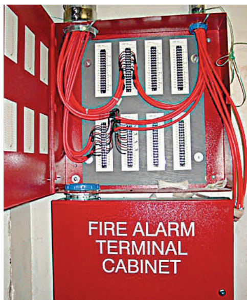
Fire Alarm Terminal Cabinet. (Source: JENSEN HUGHES, Warwick, RI)
