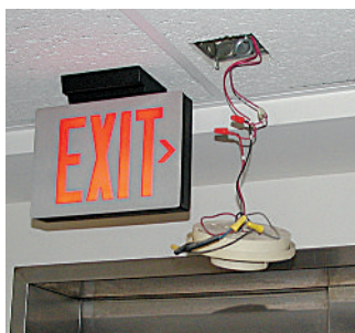
Smoke Detector Improperly Secured. (Courtesy of Jeffrey Moore, P.E., JENSEN HUGHES)
