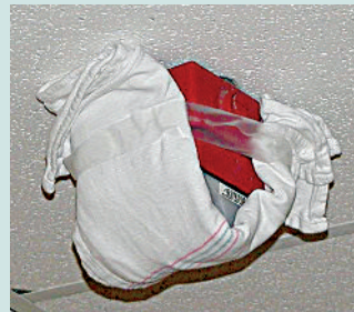
Evidence of Appliance Tampering. (Courtesy of Jeffrey Moore, P.E., JENSEN HUGHES)
