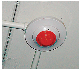
Smoke Detector with Cover Not Removed after Construction. (Courtesy of Jeffrey Moore, P.E., JENSEN HUGHES)
