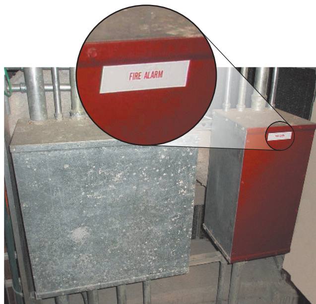
Red Box Cover with "FIRE ALARM" Label. (Source: JENSEN HUGHES, Warwick, RI)
