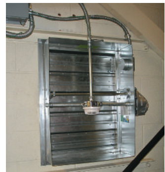
Fire/Smoke Damper Installation. (Courtesy of Jeffrey Moore, P.E., JENSEN HUGHES)
