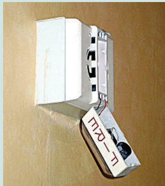
Damaged Appliance. (Courtesy of Jeffrey Moore, P.E., JENSEN HUGHES)
