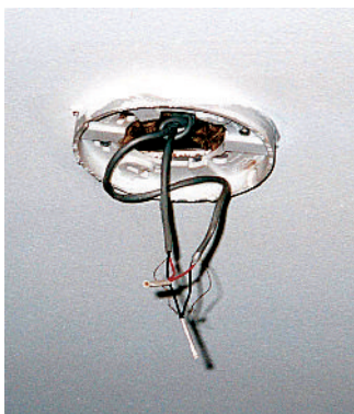
Installation with Missing Detector. (Courtesy of Jeffrey Moore, P.E., JENSEN HUGHES)
