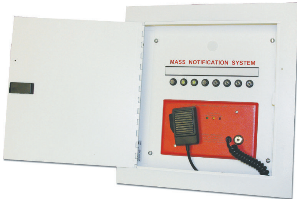
Local Operating Console (LOC). (Source: Eaton, Long Branch, NJ)
