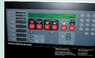
Visual Inspection of Control Unit. (Courtesy of Jeffrey Moore, P.E., JENSEN HUGHES)
