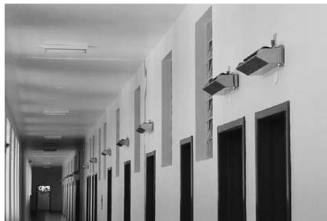
Fig. 8 Upper-Air UVC Devices in Naturally Ventilated Corridor of TB Facility in Brazil (Centers for Disease Control and Prevention)
