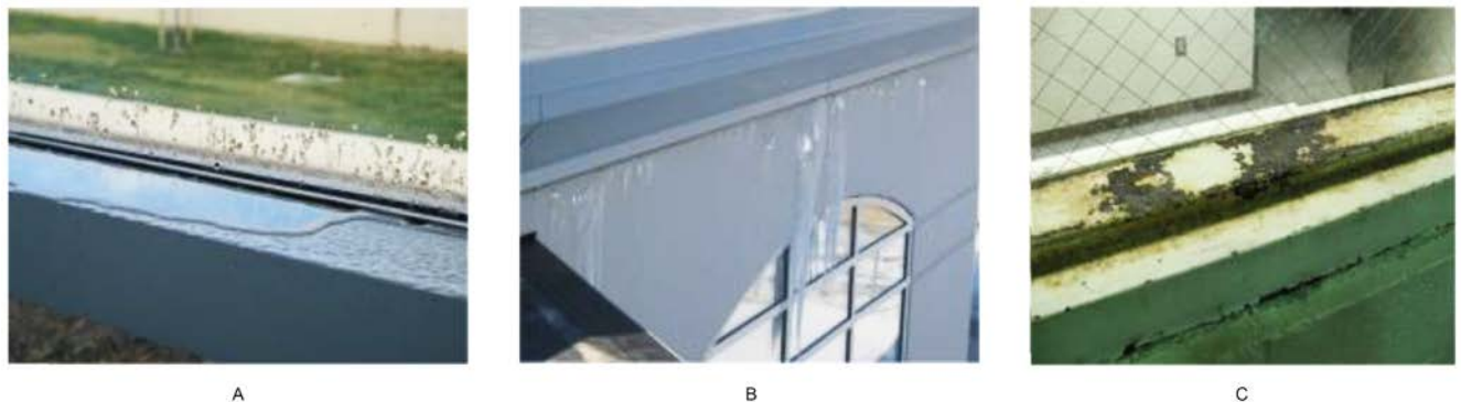
Fig. 3 Structural Damage Caused by Condensation (Courtesy Desert-Aire Corp)
