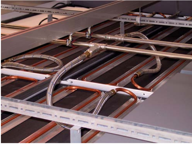
Fig. 3 Back View of Drop Ceiling: Piping Configuration with Flexible Hose and Quick-Connect Fittings
